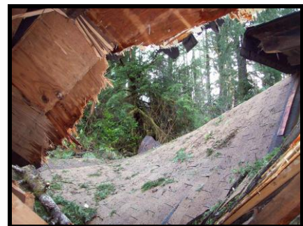
Here we're standing inside looking up toward the ceiling. Oops, big hole... and "What's that roof doing there?"
