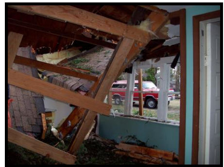
Looking out front...note the shingled roof hanging down.
